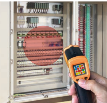
Transformers & distribution boards
